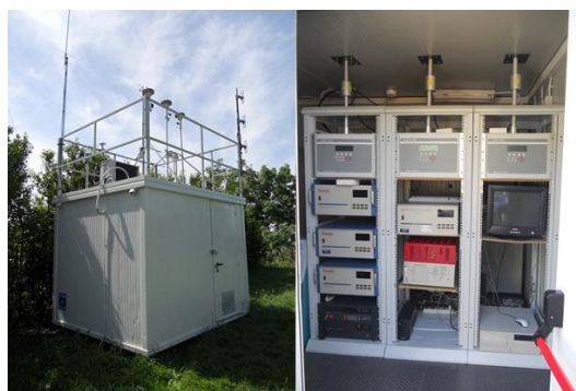
Figure 5. Pictures of the reference station in the city of Ancona.
