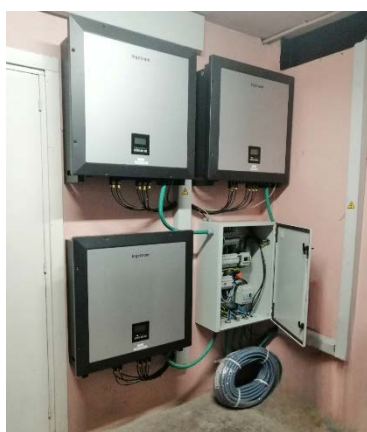
Fig. 3. Inverters of the photovoltaic installation at the DRH
