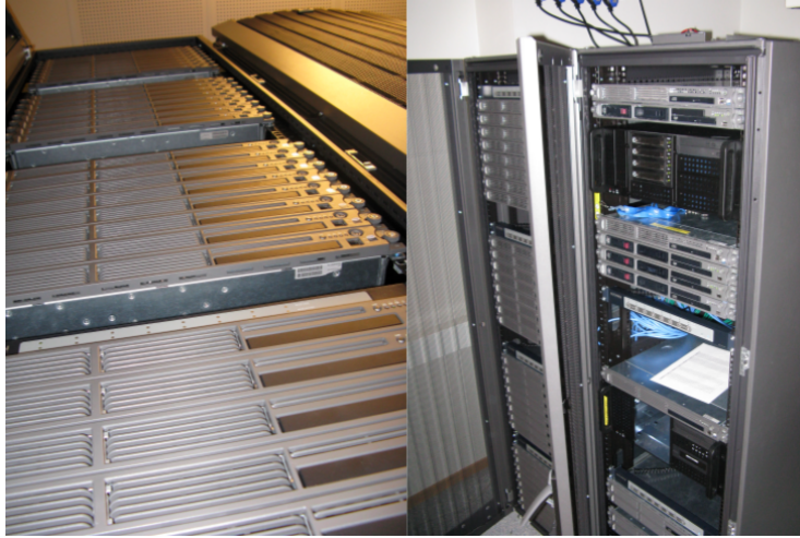
Figure 2.21: Servers of the BTH OpenLabs Security Lab
